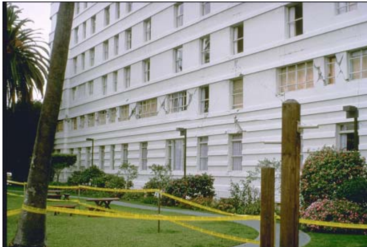
An offset from the top to the bottom of a wall, beyond what may have existed prior to the earthquake, 1" or more, may indicate severe structural damage.
